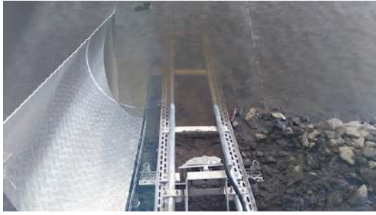
(a) The hydroacoustic velocity meter submerged.
